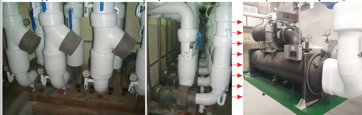
3. Actual applications of EVERGUSH CP pumps~Water supply for spa equipment
