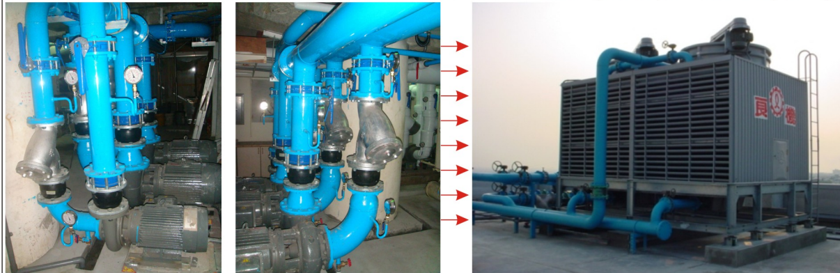
1. Actual applications of EVERGUSH CP pumps~Water circulation for Cooling Tower(air-condition systems)
